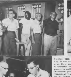
AMONG THE many tests conducted Aug. 29 was one that proves out interlocks. These are devices which prevent an operation from occurring out of sequence. In addition to Lago and Aruba Government personnel, a manufacturer's representative also observed the switching. Mr. Osborn and Mr. Gaba constantly referred to meter readings to assure correct positioning and synchronization. ENTRE E hops testnan conduci Aug. 29 tabata uno cu ta stima cramentoso. Esakinan ta aparatonan cu ta preveni un operacion di sucede for di su ora. Fuera di personal di Lago y gobierno, un representante di e fabrica tambe tabata observa e switchmento.
